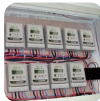
Power Distribution Panels
